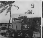
The problem of how to supply power was ingeniously solved when C&I set up a winding generator. Residents must be careful, not to use too much electricity at one time.
